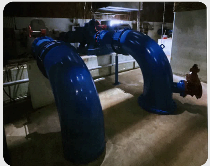
Backwash pumps installed at the Vicksburg Water Plant
